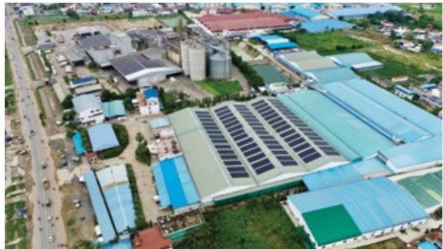
Vanco Rooftop Solar PV Project - completed in 2022
