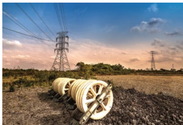
North Phnom Penh – Kampong Cham Project – completed in 2013
