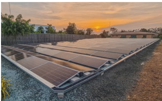
Kboun Village Rooftop and Ground-Mounted Solar PV Project - completed in 2023
